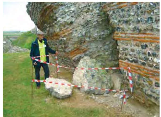
The dislodged section of Roman masonry at Burgh Castle.
