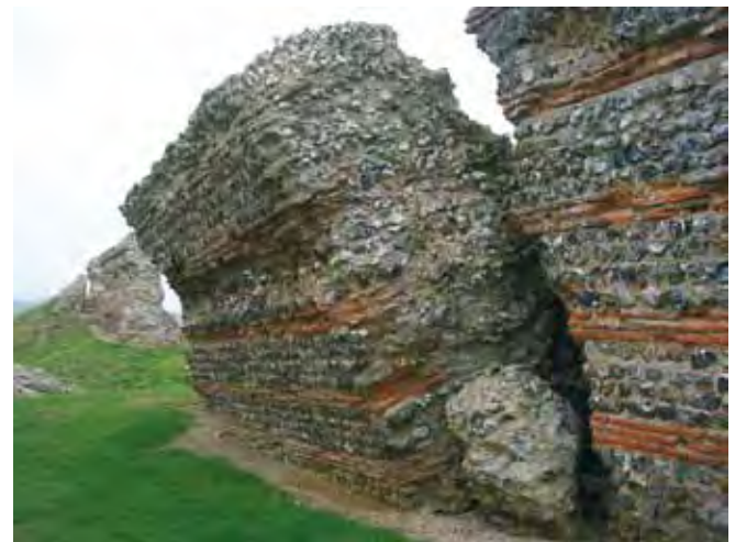
The leaning section of the south wall at Burgh Castle with the lump of Roman masonry to the right which has recently been dislodged, probably through vandalism. Photo by David Gurney.
