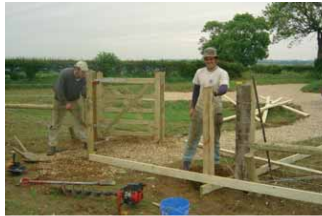
Construction of disabled access kissing gate at the new car park at Bloodgate Hill, June 2004. Photo Peter Wade-Martins
