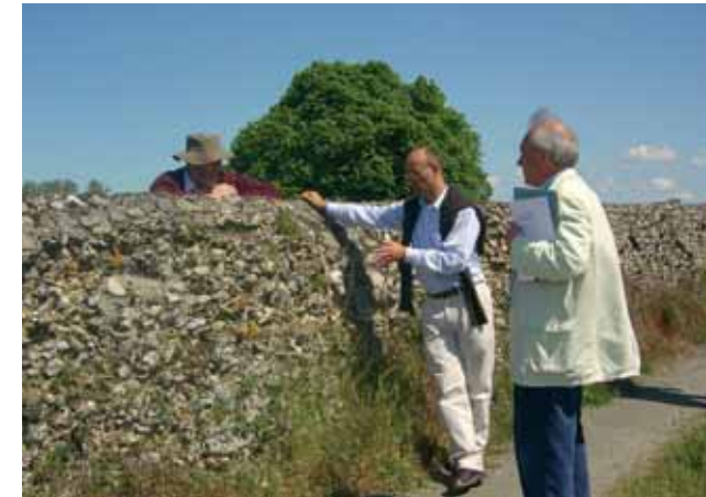
A meeting in May 2004 with English Heritage representatives Michael Wingate (left) and John Ette (centre) and Stephen Heywood, historic buildings advisor to the Trust, to discuss in detail how best to repair the crumbling medieval precinct wall which the Trust has recently purchased as a conservation measure. Photo Peter Wade-Martins
