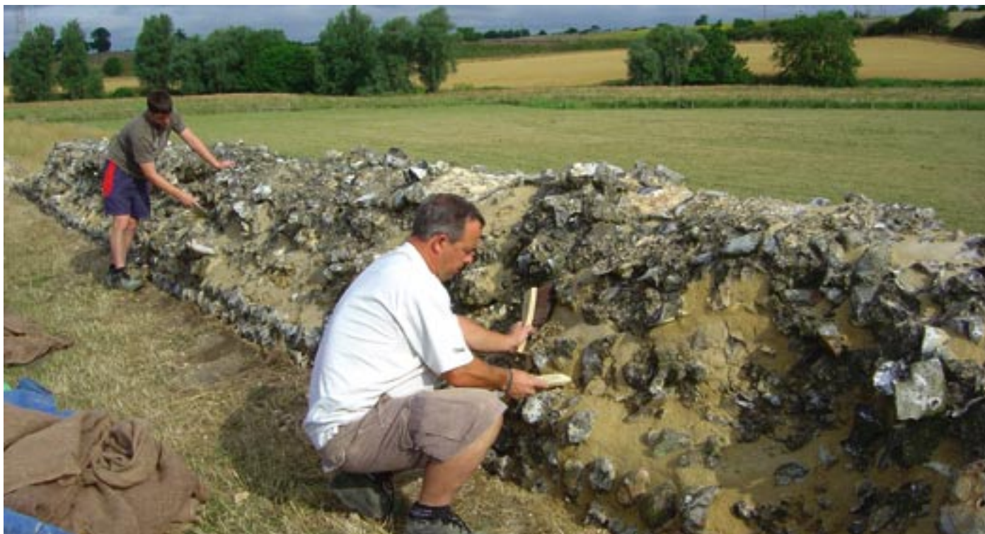
Adrian Fox, foreman of the team working at Caistor, brushing down a fresh area of mortar on the inside face of the north wall. Photo Peter Wade-Martins
