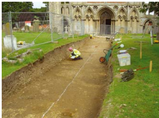
Excavations in advance of the new Binham church path revealed ditches and other features pre-dating the burial ground.
