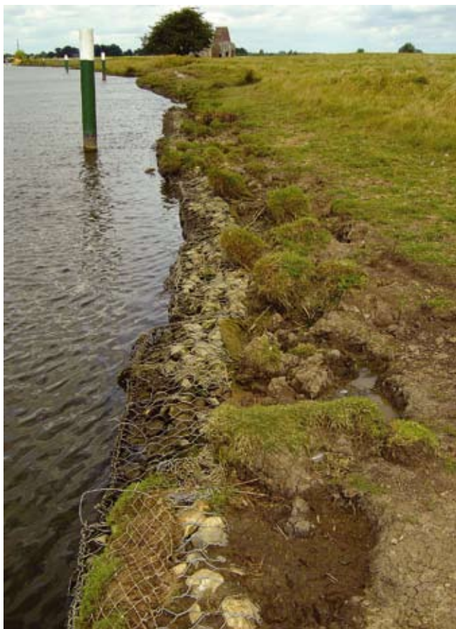
Erosion of the riverbank caused by high water levels and cattle trampling have exposed the stone-filled wire gabions. Further work is now urgently needed to make the gabion tops safe to walk on.
