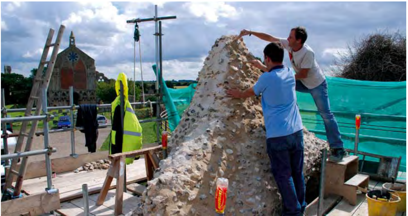
Topping out the rough racking on the gatehouse at Binham with the priory church behind.
