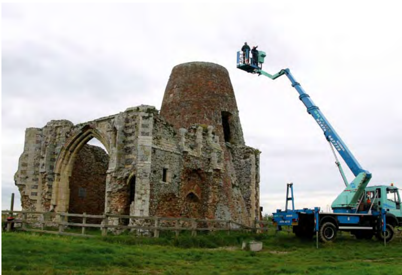
High level inspection of the gatehouse and windmill in September showed that while repairs were needed, there were no major defects.
