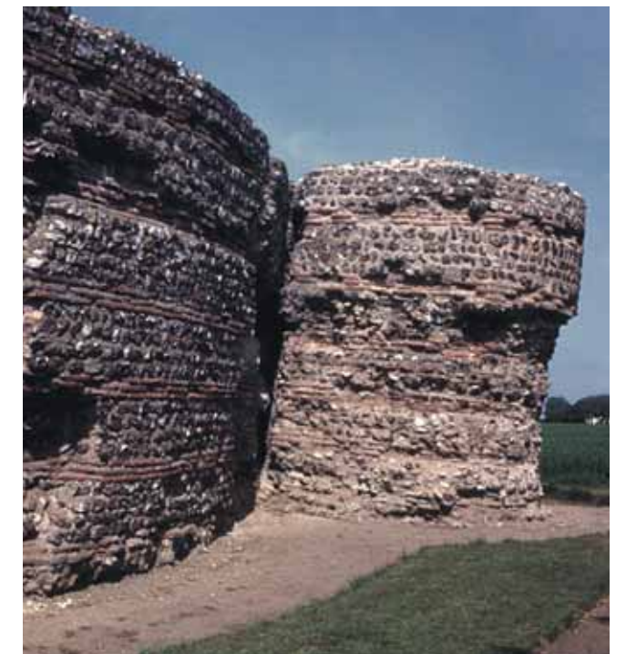
Part of the south wall and the south-east bastion of the Roman fort at Burgh Castle. A nineteenth-century engraving of this bastion is now the Trust's logo.
