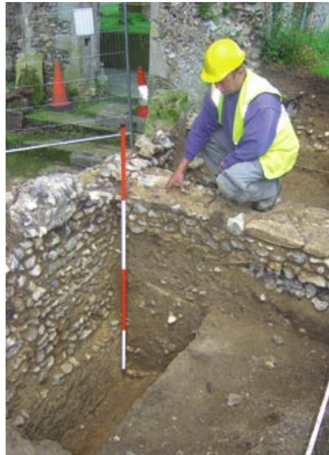
The Norman foundations of the north wall proved to be massive, well able to support the modern structure to be placed upon it. Photo Peter Wade-Martins
