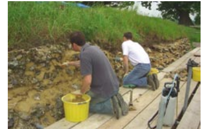
Work on re-pointing the Roman flintwork in progress. The mortar is placed so that it slopes down to shed water from the wall, thus reducing frost damage. Photo Peter Wade-Martins
