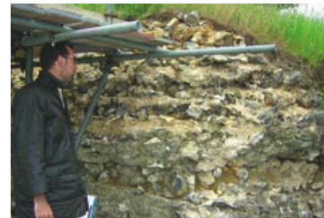
The horizontal layering or "day lifts" in the Roman wall construction has become evident as the wall has been cleaned down prior to re-pointing. Photo Peter Wade-Martins
