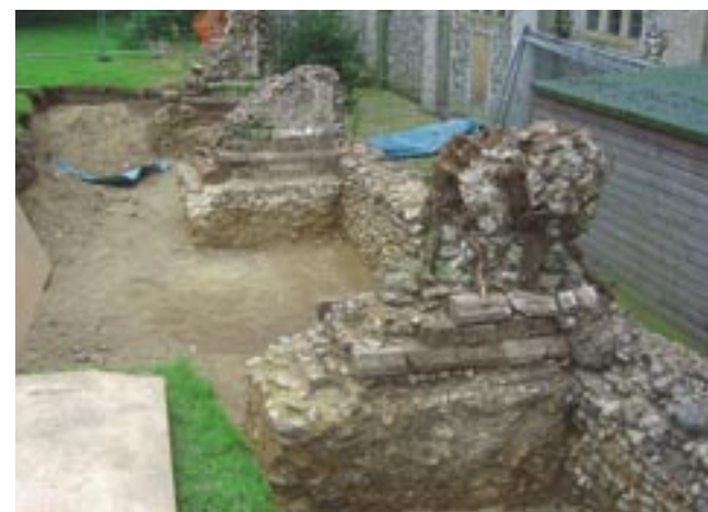
Excavation of the north aisle of Binham Priory church, by Archaeology Project Services of Lincolnshire, was designed to expose the north wall and buttresses. The church community intend to use the first four bays of the aisle to create a new church entrance, display area and toilets. Photo Peter Wade-Martins
