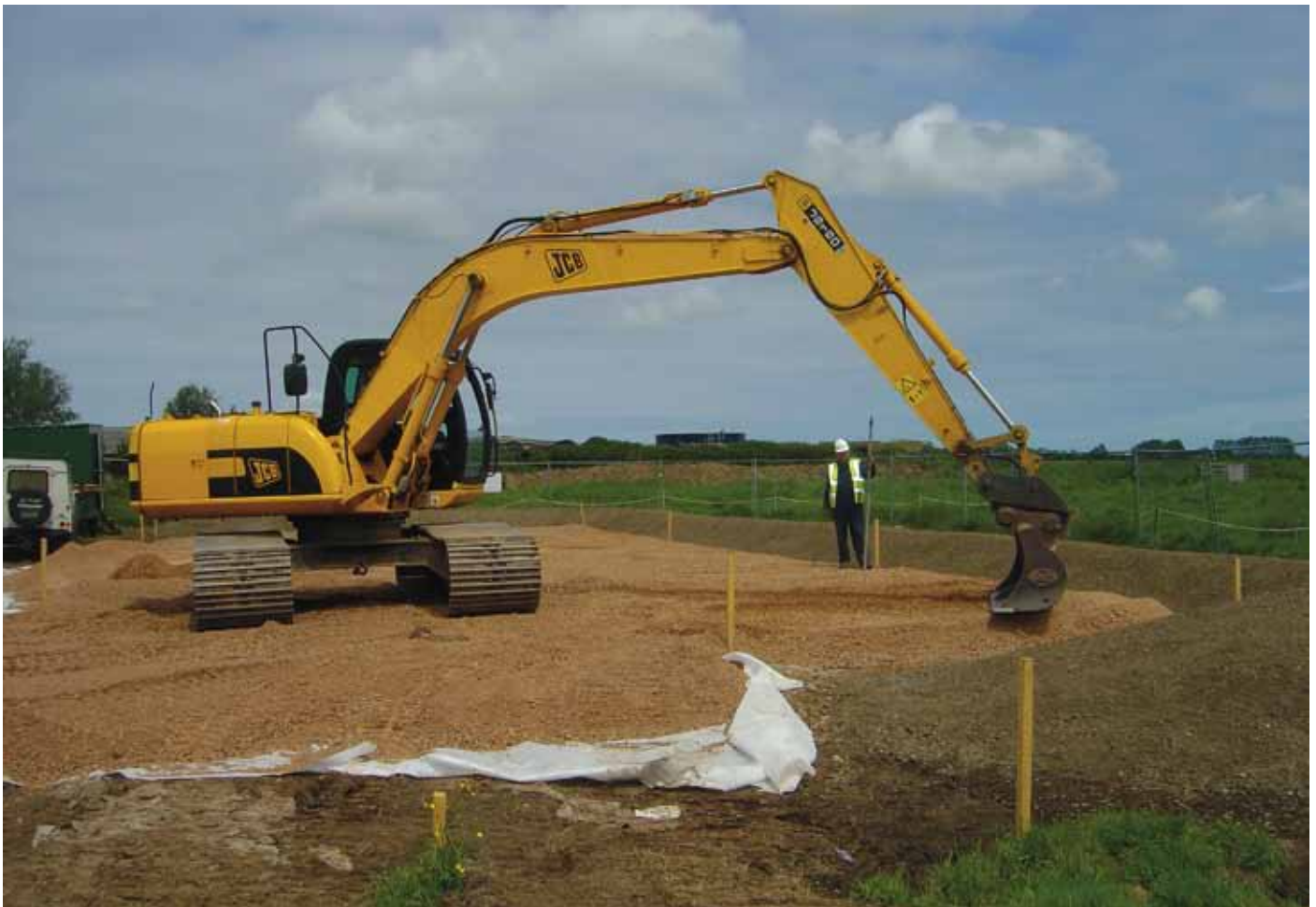
The construction of the new car park for St Benets Abbey is being run by a Broads Authority work team who are acting as contractors. The hard standing created using crushed stone was surrounded by a low earth bank. Over the crushed stone a layer of sand has been laid to form a bedding for plastic “Ecoblocks” to be filled with soil and grass seed to form a green hard standing for cars.
