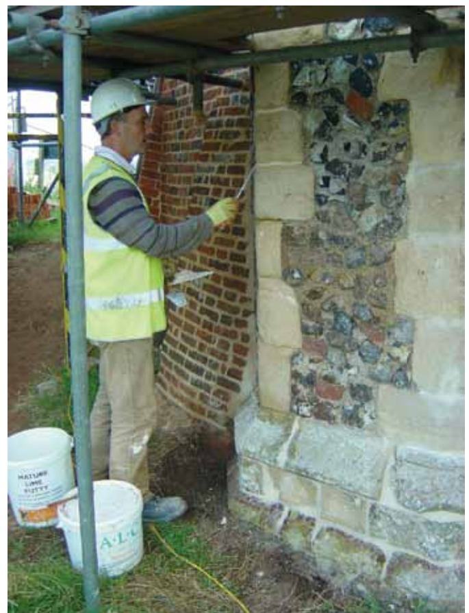
Most of the stonework in the gatehouse was in good order and the joints were just raked out and filled with fresh lime mortar.
