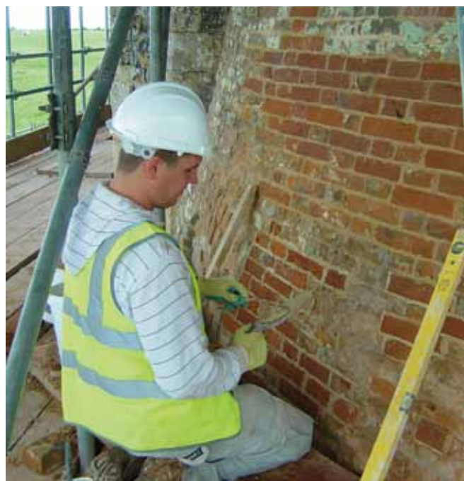
Three thousand five hundred and fifty bricks were cut out from the windmill and replaced with matching hand-made replacements from the Bulmer Brick and Tile Company in Sudbury. Our contractors have calculated that a total of 960,000 bricks were originally used to build the windmill.
