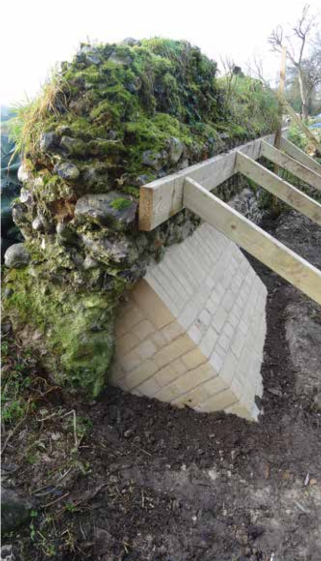
Fig 6: Burnham Norton. New buttress installed to support the standing section of north wall.
